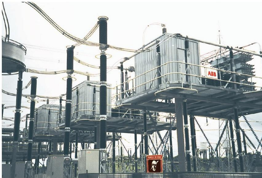
Figure 3.1 -Transmission Line Series ABB TCSC on Platform [16]
