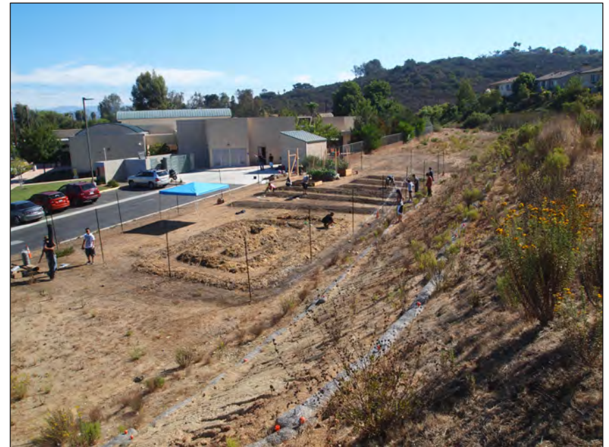
Figure 4.—In this photo from October 2012, students are installing the garden's first deer fence. Today the garden has a larger footprint surrounded by a chain-link fence. Source: author
